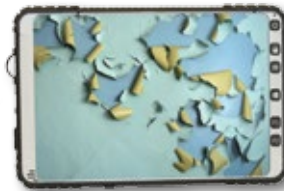
Tank lining delamination image as displayed on tablet
